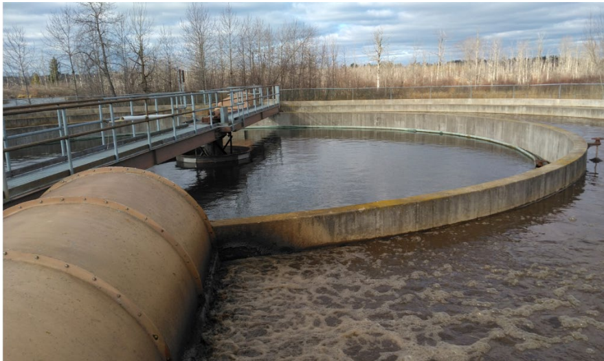
Picture 1. Secondary Clarifier
