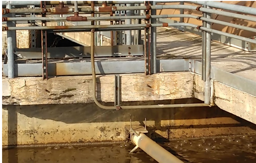
Picture 2. Secondary Clarifier Structural Damage
